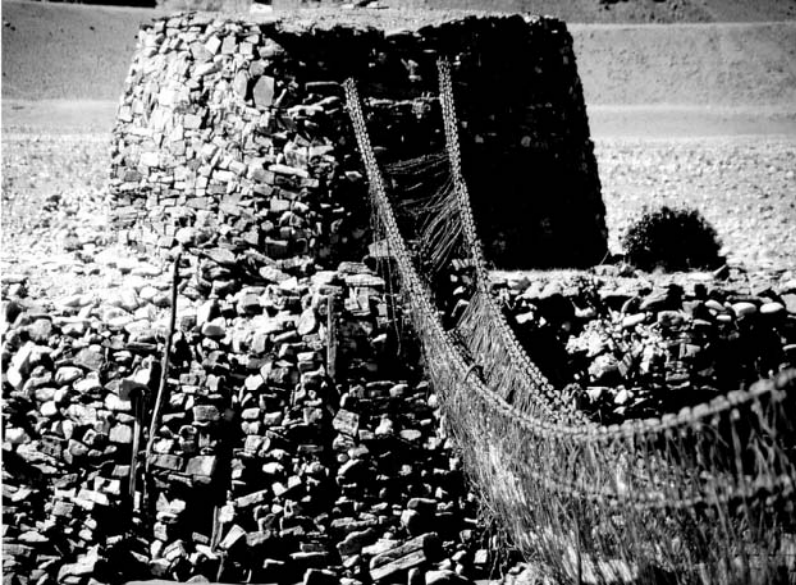
Fig. 26: The part of the Phuntsoling Chakzam across the Yarlung Tsangpo, which is still functioning.
